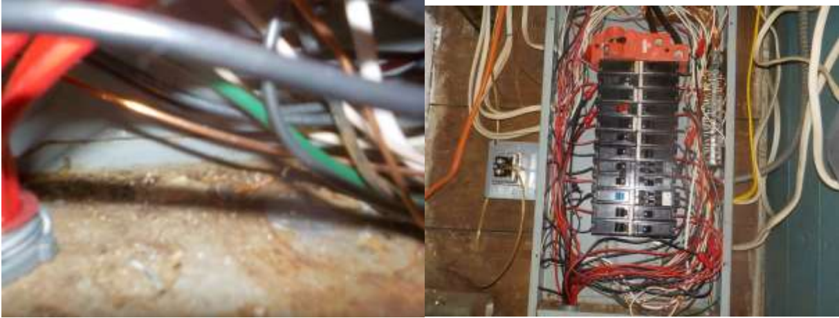
OVERALL VIEW OF PANEL, RUST, DETERIORATION, CORROSION
