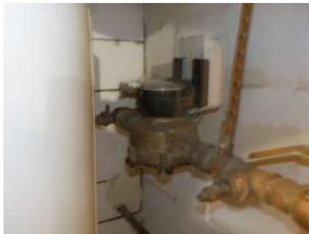
WATER METER AND MAIN WATER SHUT OFF
