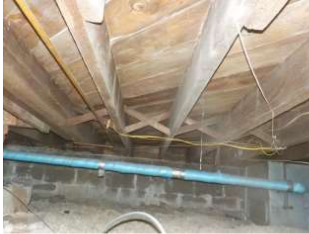
CRAWLSPACE NEEDS INSULATION AND OXIDIZED PIPES
