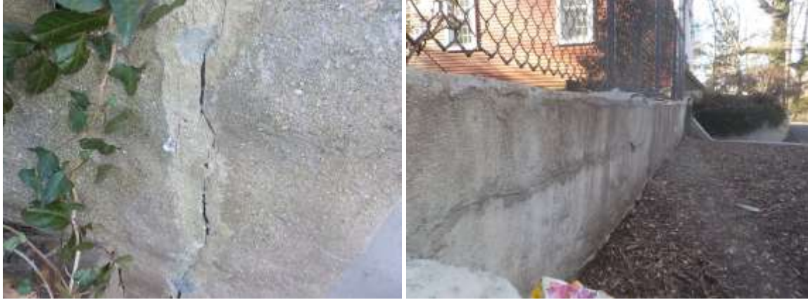
CRACKS TO RETAINING WALL
