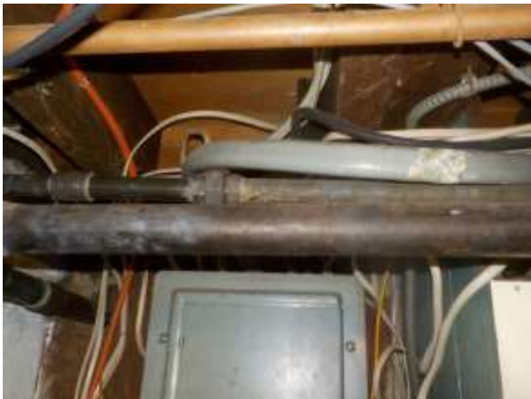
PIPES TOO CLOSE TO PANEL
