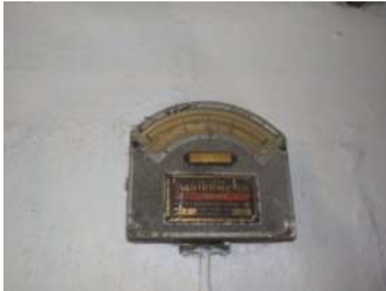
OIL TANK GAGE
