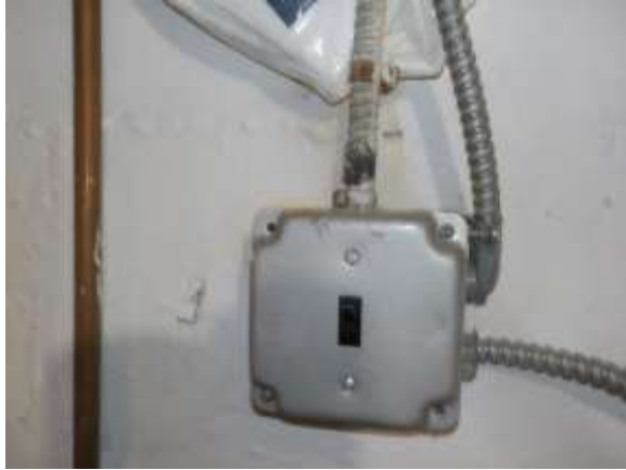
EMERGENCY SHUT OFF SWITCH
